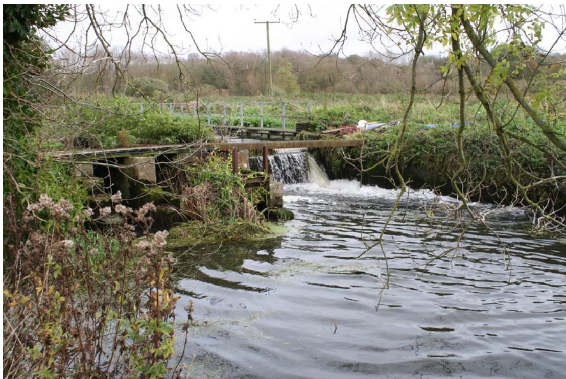
Figure 1. The structure, looking upstream. The fish farm intake is visible above the structure, with a walkway and handrail running over it. The residual flow passes mainly through a notch against the far bank, with some passing over a level board across a wide crest (centre-right of picture). The other hatches, including the eel trap (centre of picture) are closed.
