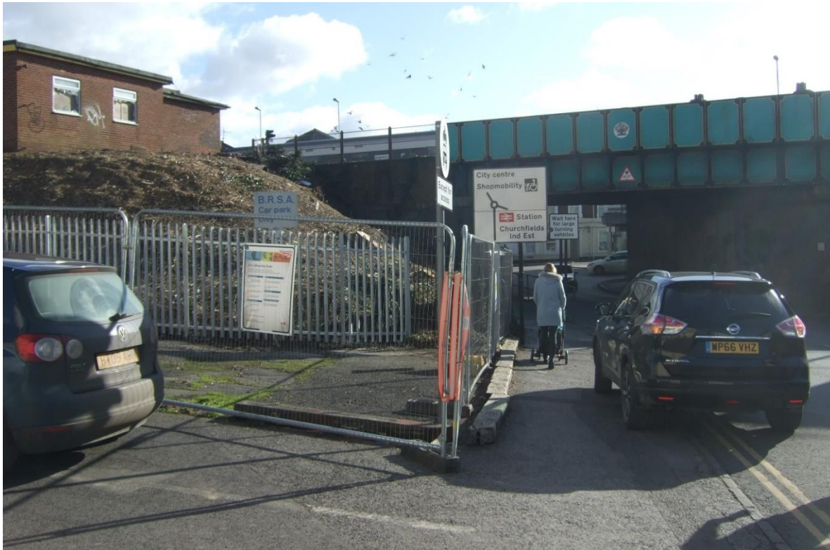
Figure 2-3 Former rail club (currently being demolished) and rail bridge over Fisherton Street
