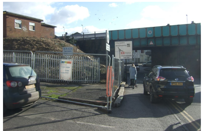
Photo 4: Former Rail Club (currently being demolished) and Rail Bridge over Fisherton Street
