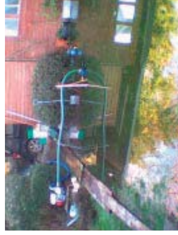
A submersible pump in operation
