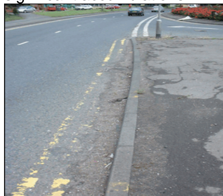
Detritus Grade D - Heavy with significant accumulations
