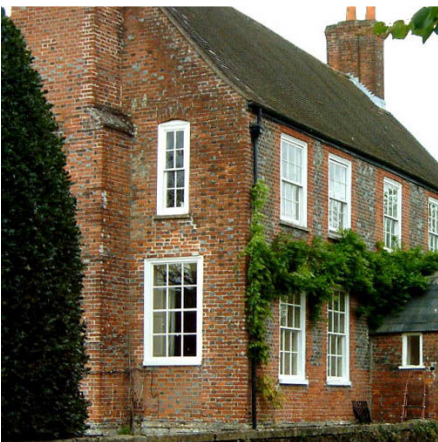
The attractive appearance of historic brickwork, as at Manor Farmhouse, results from the combination of brick colour and texture, the bond used in construction, and the lime mortar. The side windows here are a recent alteration.
