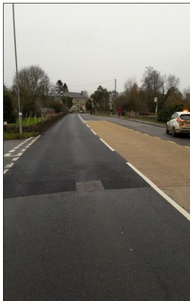
The programme of road resurfacing is improving the strength and surfaces of the county's road network.
