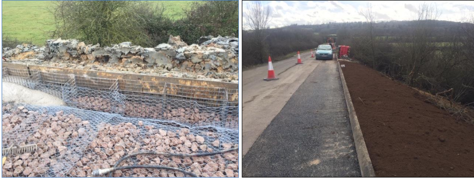
Major repairs using gabion baskets were undertaken to address serious verge and carriageway edge failure
