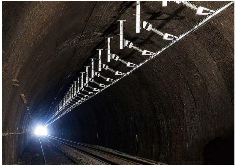
Solid Conductor Rail (SCR) within the Severn Tunnel - two of these (each 4 miles long) will be installed
