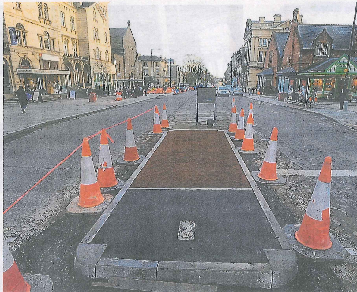
● The changes to Whiteladies Road are designed to give priority to buses and pedestrians
