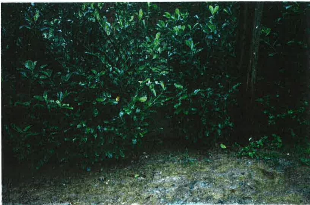
The now non-accessible telecom/broadband junction box.
