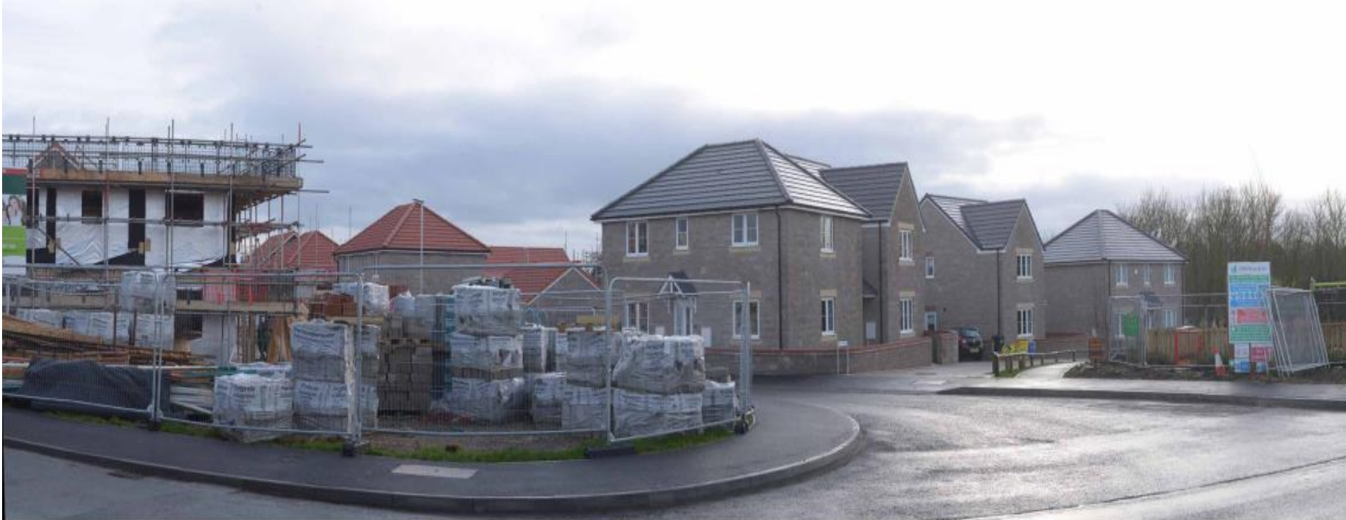
VIEWPOINT: 1 LOOKING EAST TOWARDS THE SITE FROM THE PAVEMENT ALONG RESTROP ROAD.
