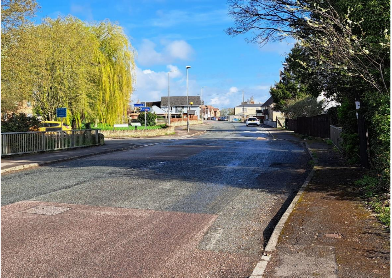
Semington Road – north of access – reconstructed lay-by to widen the existing foot path.
